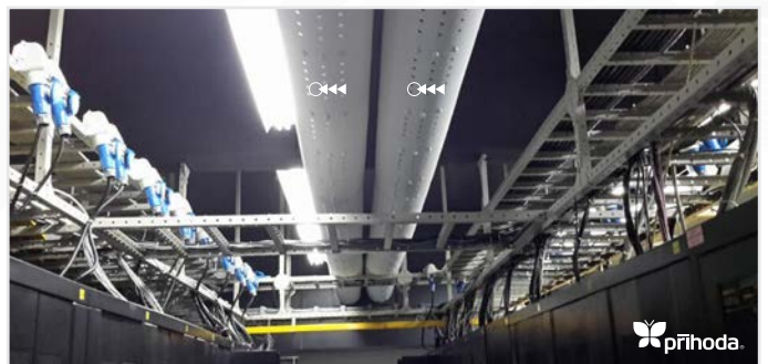
Server room, Leshan City, China
